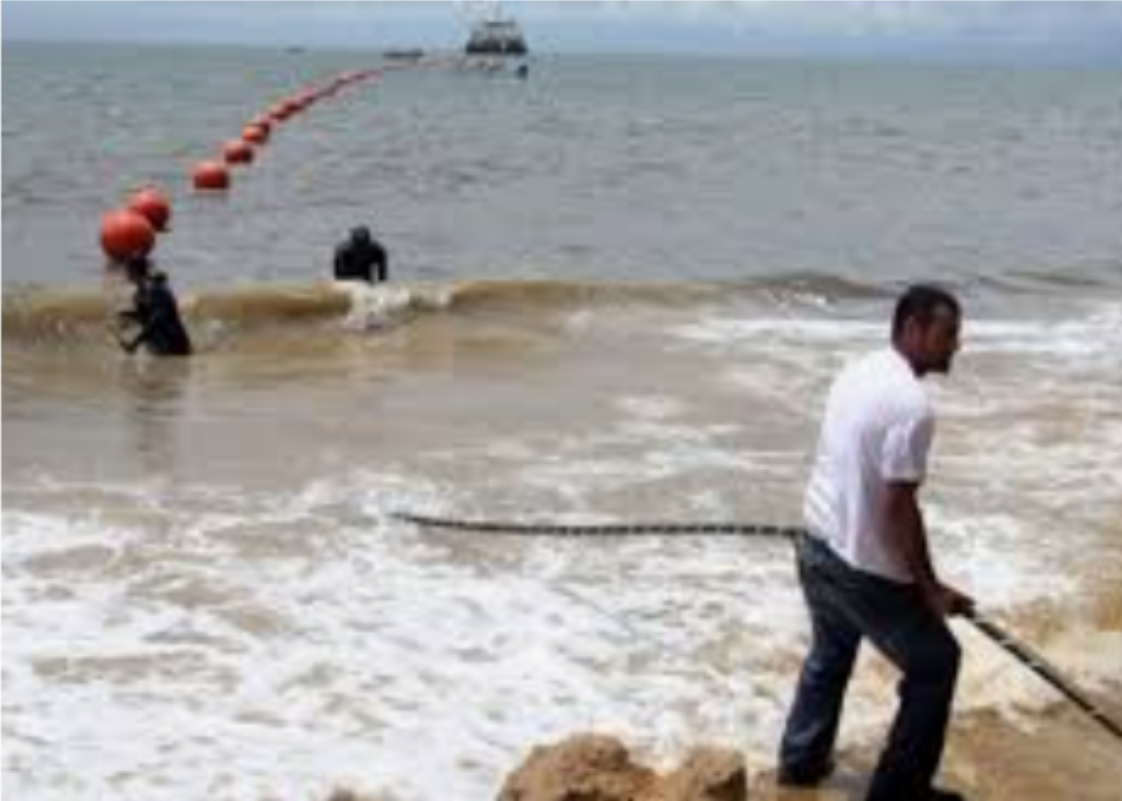
Figure 2. ACE Cable Landing in Monrovia (2011)
